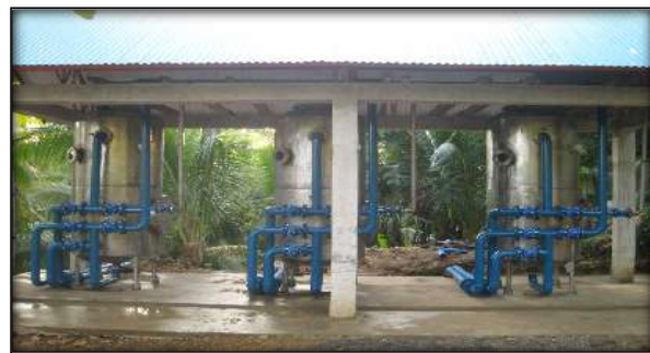
Manampa Softening Facility
