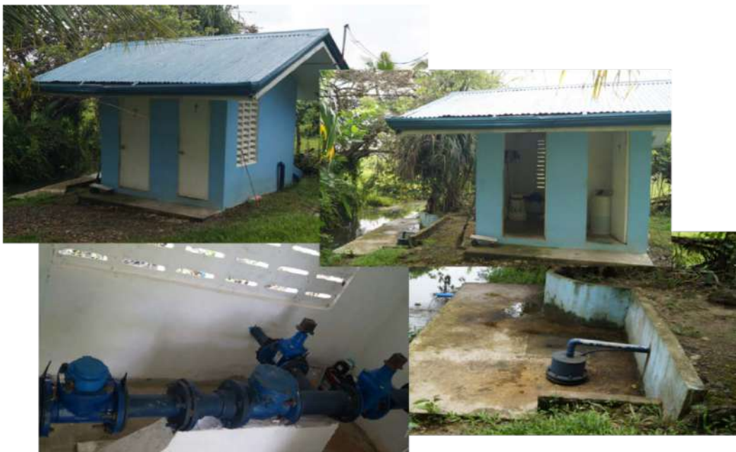
Omod spring box and pumping station.
